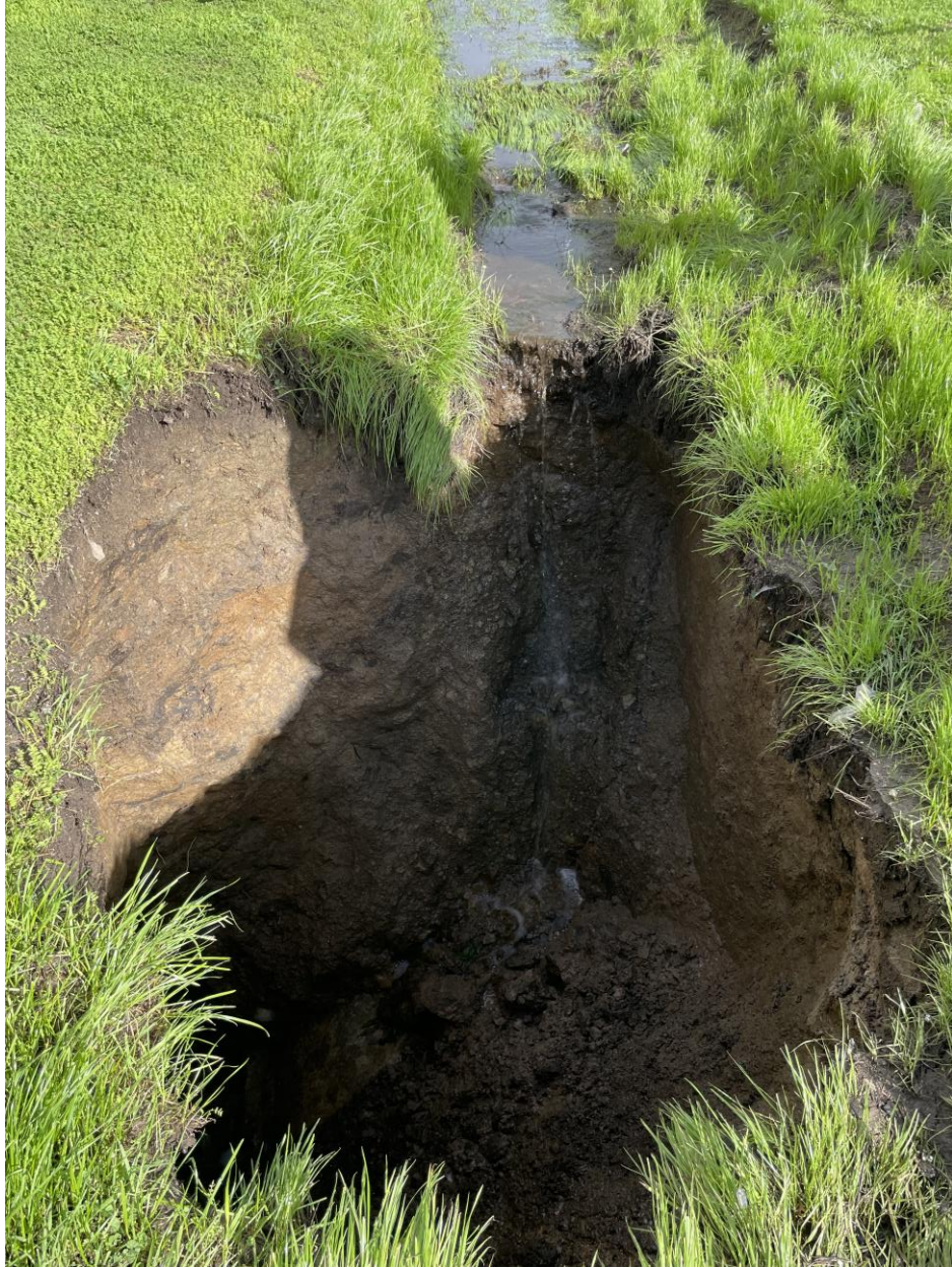
Sinkhole showing surface drainage
