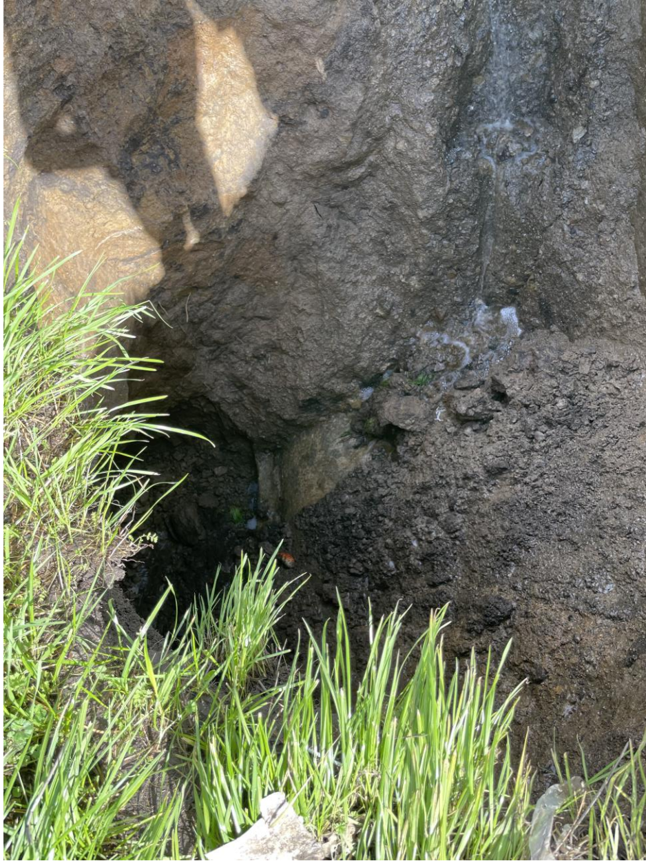
Sinkhole showing concrete pipe
