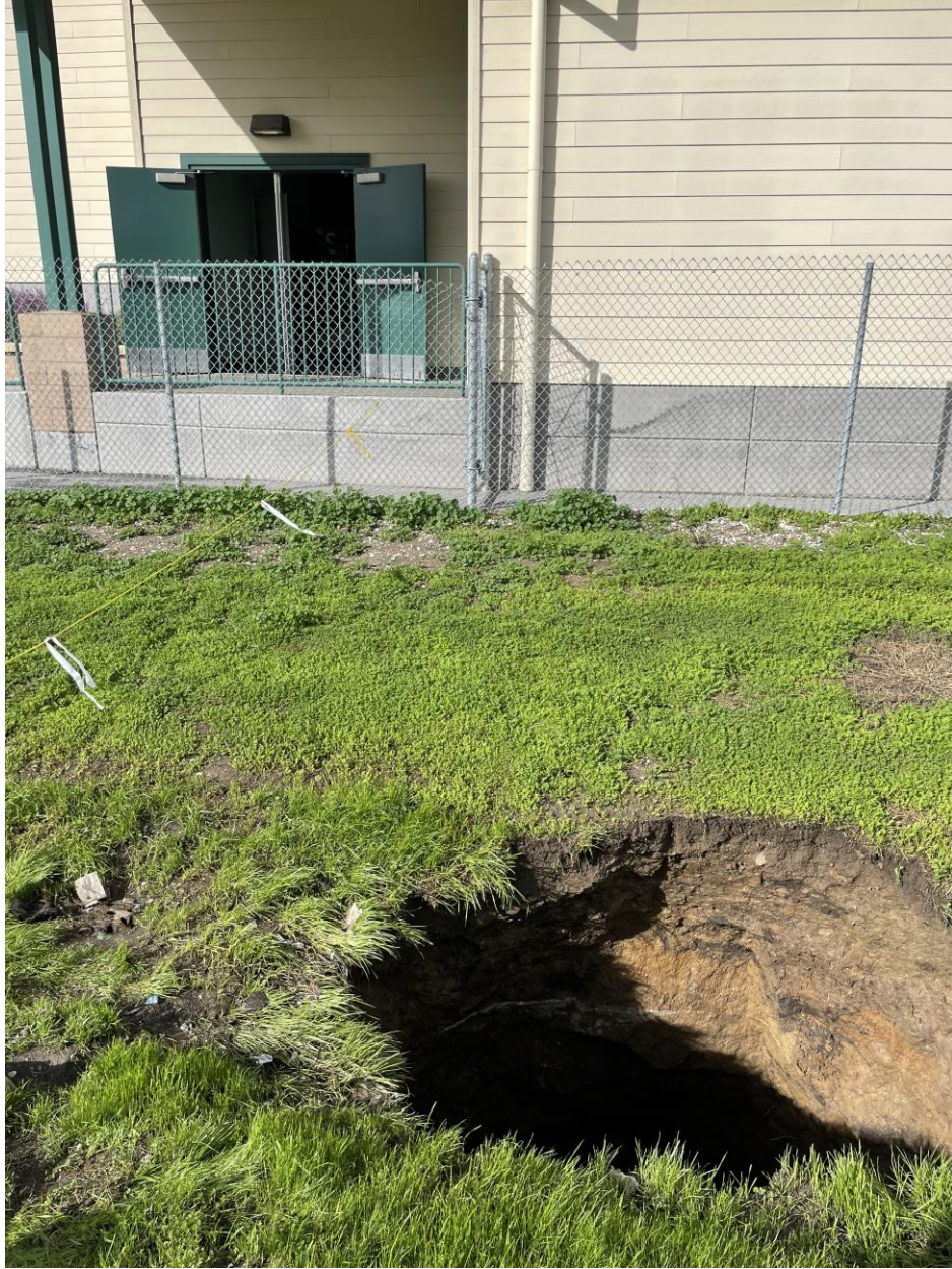
Sinkhole with Los Padres Elementary School multi-use building in the background
